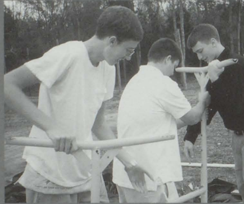
Below: Men at work... Brian Stewart, Casey Singleton, and Chase Middleton use their bulging muscles to lift equipment at the girls softball field.
