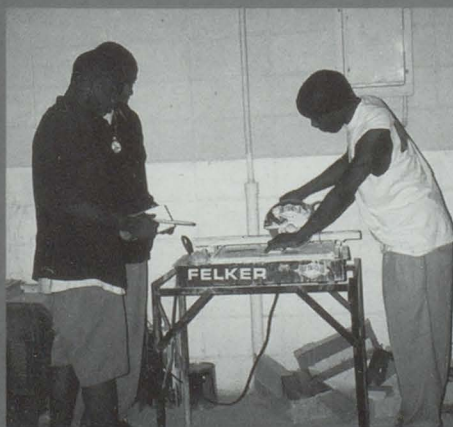
Above: Workin' Hard... Masonry students are working together to cut ceramic tiles.
